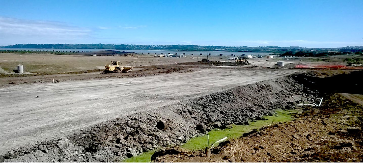
Under construction – looking north, an embankment for a new link road to Puketutu Island, mid February 2014.
